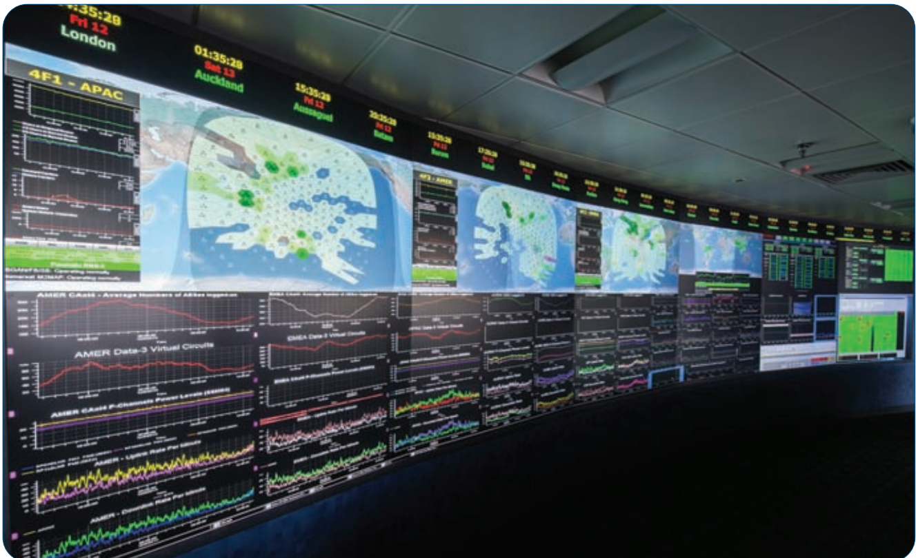
Inmarsat network operations centre
